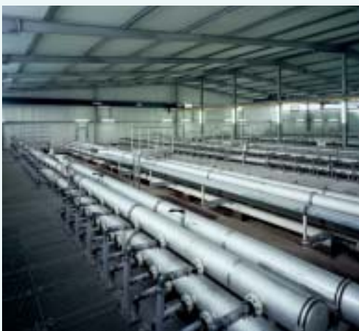
Membrane activation tanks at Erftverband's Nordkanal treatment plant.
